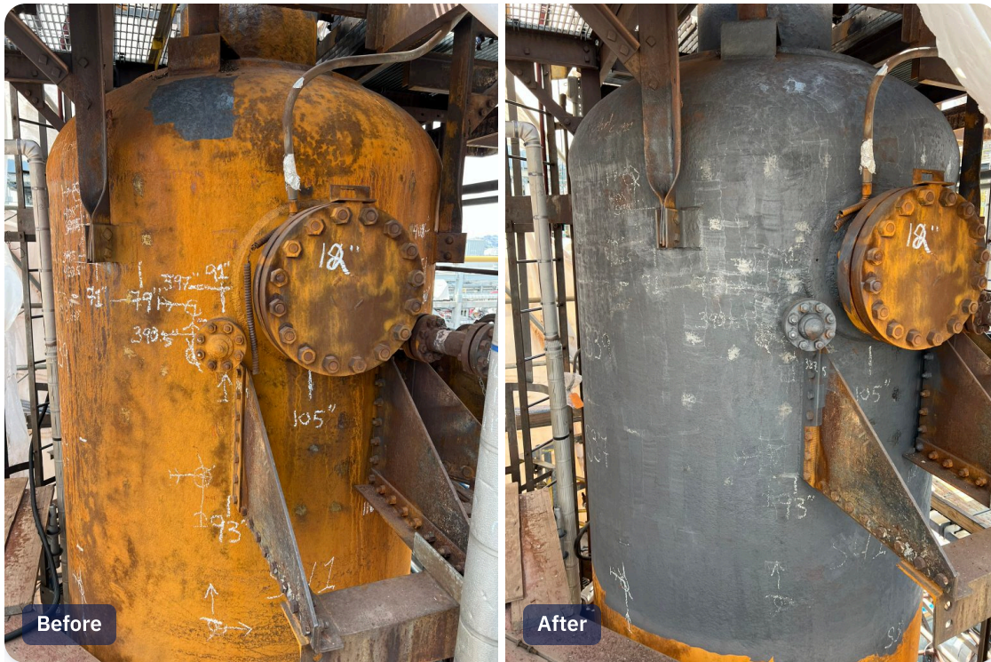
Process vessel and 12 in manway
